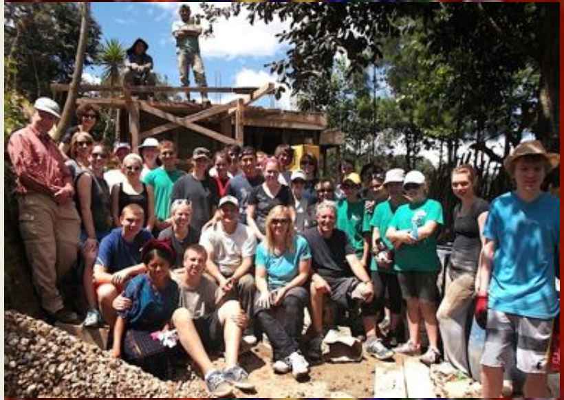
(Above) Team Internat'l Co-op helped pour the concrete roof (la terraza) at Eusebia's family house in Xolbe. Bruce Izard is seated, front row, at center, in black shirt.
